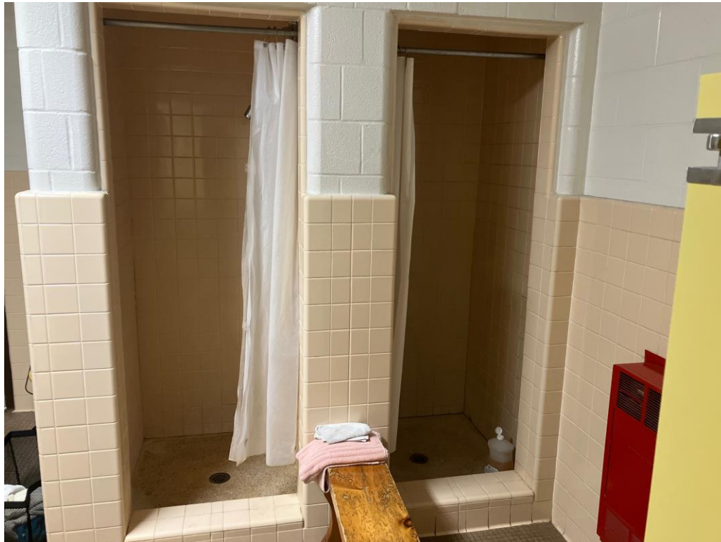
Lack of privacy in showering areas
